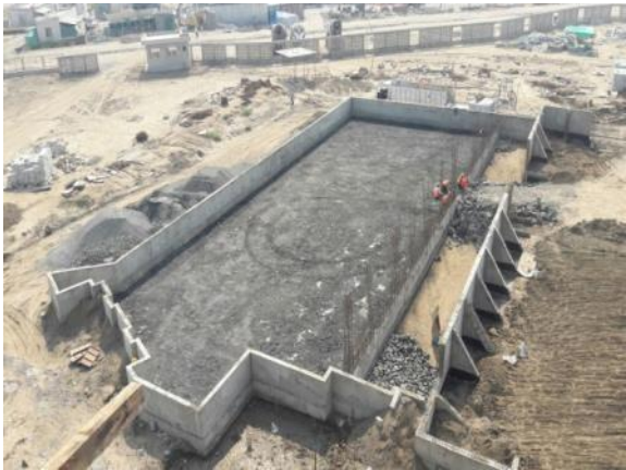
Reflecting pool – Rubble soiling
